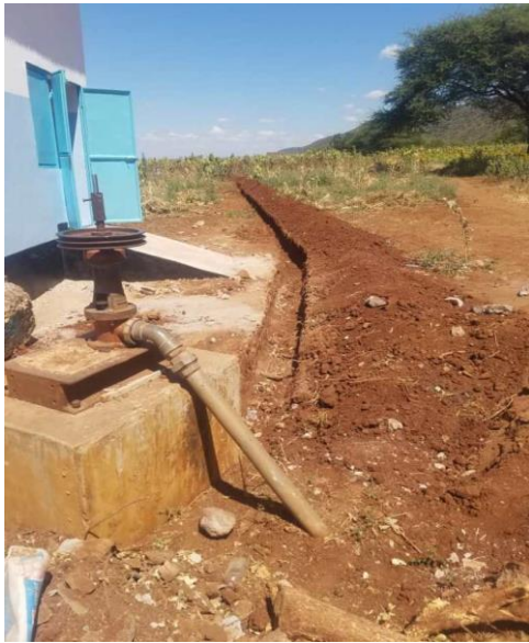
New water pump installed
