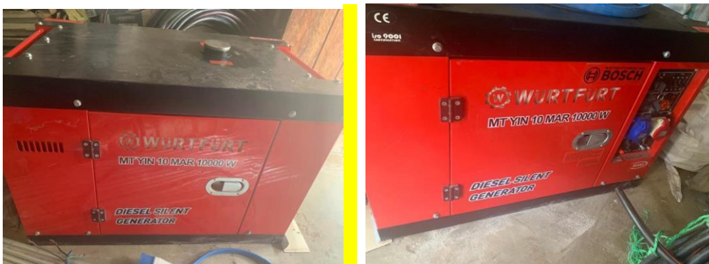
Generator for power supply
